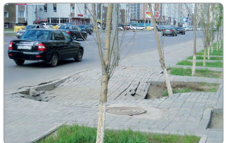
Subsidence in urban area induced by water network leakage. Credits: meadowsaffron on flickr
